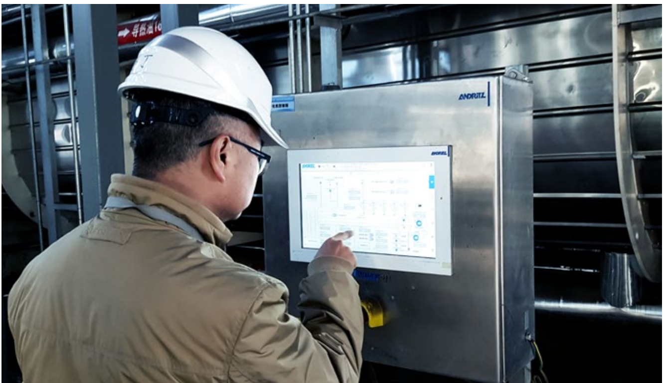
Automated operation systems
